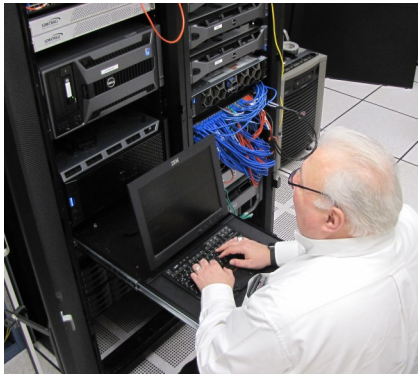
RCLS Computer Room
