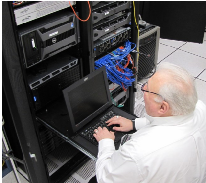
RCLS Computer Room
