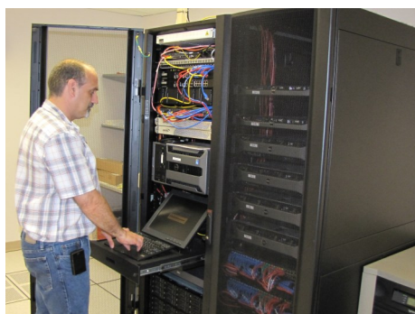
RCLS Computer Room
