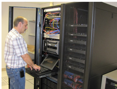
RCLS Computer Room
